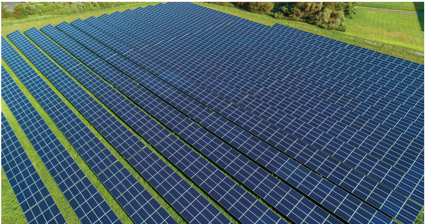
Ground-mounted solar at the Estee Lauder Companies’ campus in Melville, NY. © EmPower Solar
