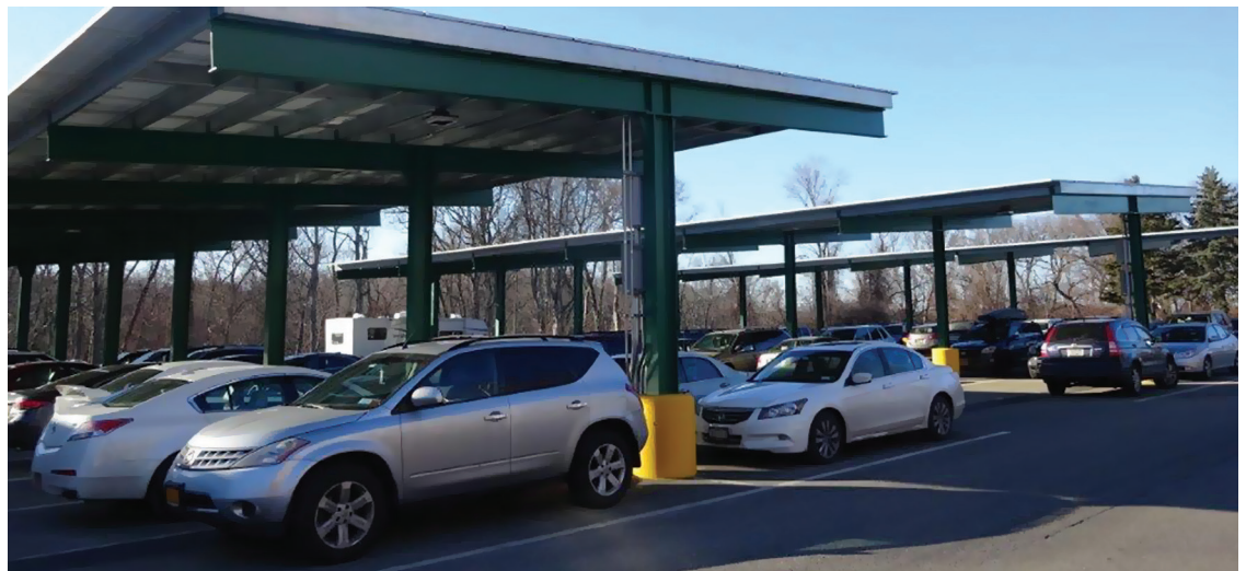
Solar canopies cover parking at the Northport VA Medical Center. © Sunshine Plus Solar
