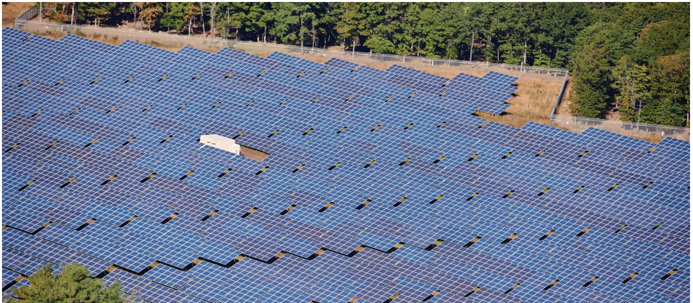
The 32 MW Long Island Solar Farm at Brookhaven National Laboratory was built through a collaboration between BP Solar, the Long Island Power Authority, and the U.S. Department of Energy. © Flickr
